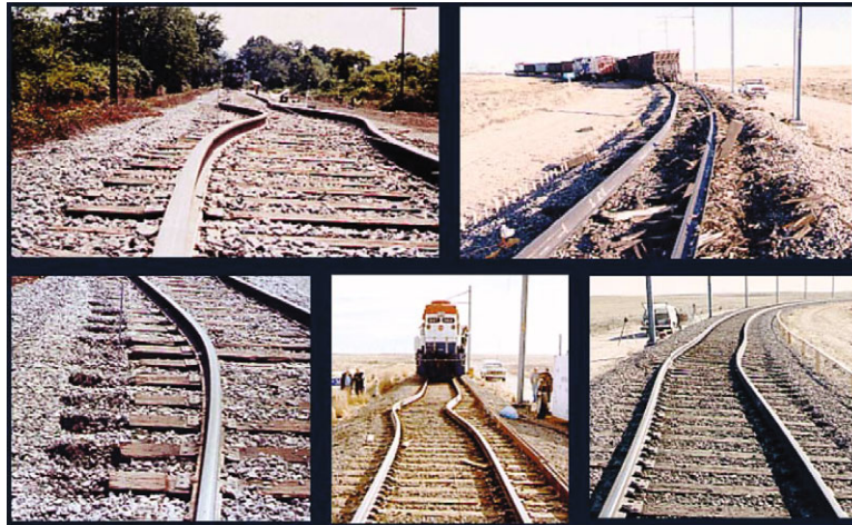
Figure 1.4: Thermal buckling of railway rails, also called “sun-kinks” (photo courtesy of Volpe, The National Transportation Systems Center, USDOT).
